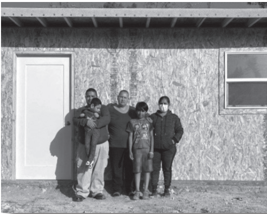
From left to right: Alberto, Edgar, Doris, Jose and Maria. They haven't decided yet if they want to paint or if stucco would be better. Either way they're happy to be in!
